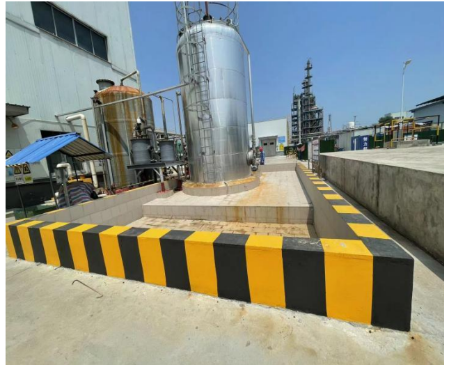
废液收集池及围堰
